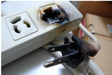
Incomplete insertion of a plug
