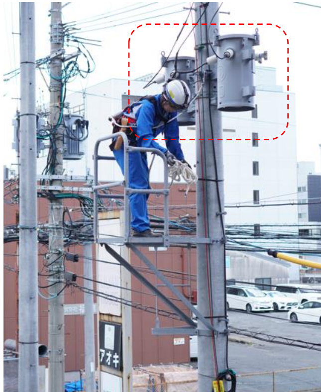
[Demand equipment installed on an electric pole]
