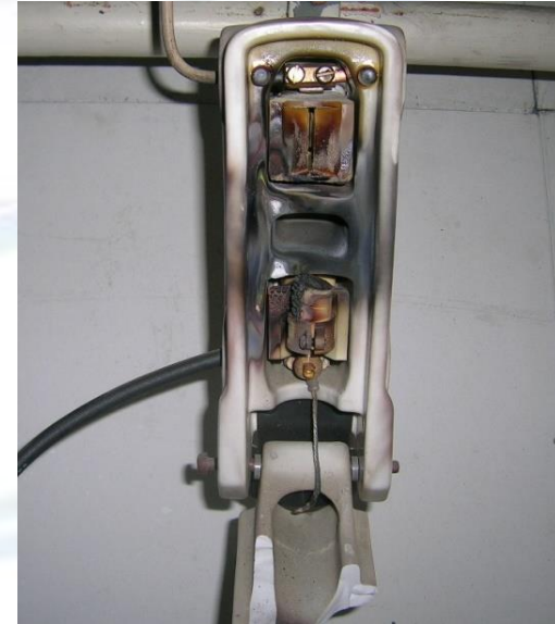
Fuse burnout due to degradation over time
