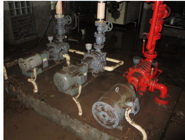
[Motors damaged by a flood]
