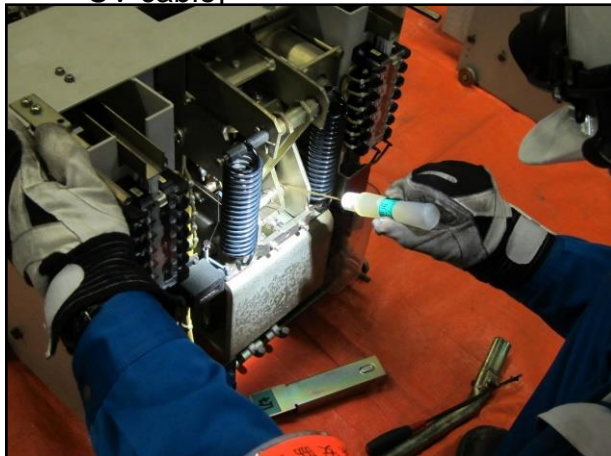
[Maintenance of a circuit breaker] fisuel seminar – 15 and 16 October 2024
