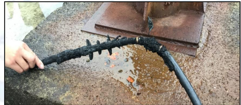
high voltage CV cable electrical breakdown (burnout)
