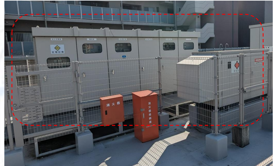
[Demand equipment in a common tenant building (8 story)]
