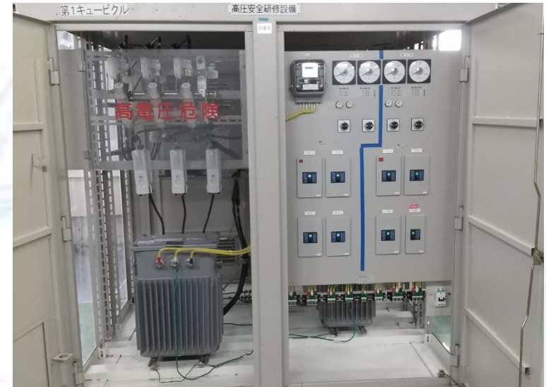
[Demand equipment of the cubicle type (front)]
