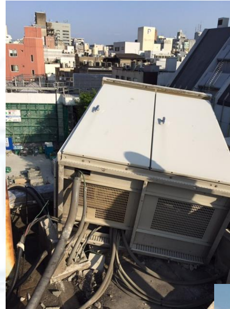
[Substation equipment damaged by an earthquake]
