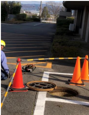
State of the lid of the manhole being laid upside down
